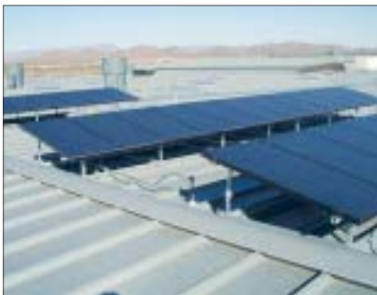
Rooftop photovoltaic array that collects energy during the day helps to power parking area and other outside lights at night.
