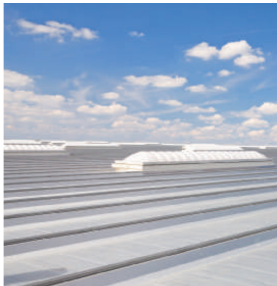
A total of 70 SunLite Strip™ daylighting system units provide nearly 30 foot-candles of natural light into the manufacturing space.
